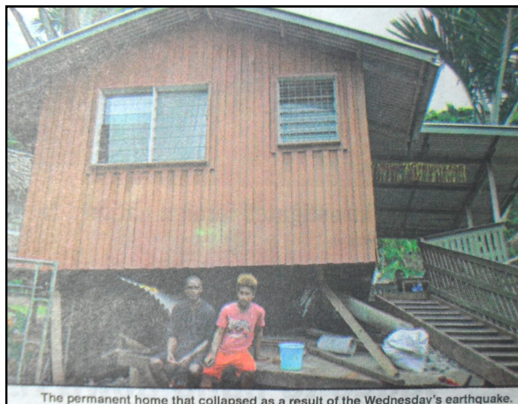
The permanent home that collapsed as a result of the Wednesday's earthquake.
